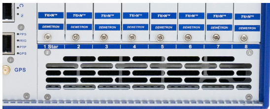
Fig. 17: Intake vents with filter pads
